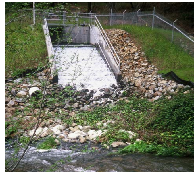
Grass Valley's effluent discharge to Wolf Creek via a cascade aerator.
