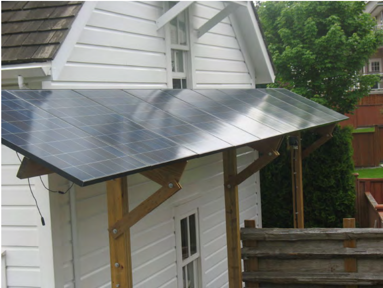
Solar panels installed properly on a historic property. Note the separation between the rear of the home and the solar panels affixed to structural columns.
